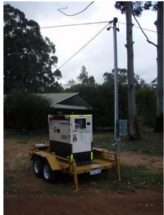
Power is being temporarily maintained by a generator
